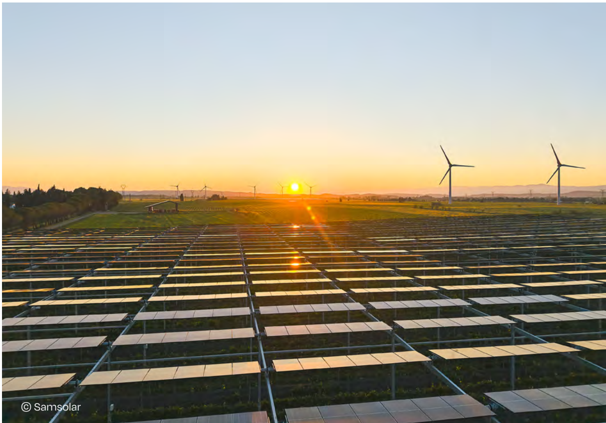
© Samsolar 3 MW Agri-PV plant in Cruscades, France.
