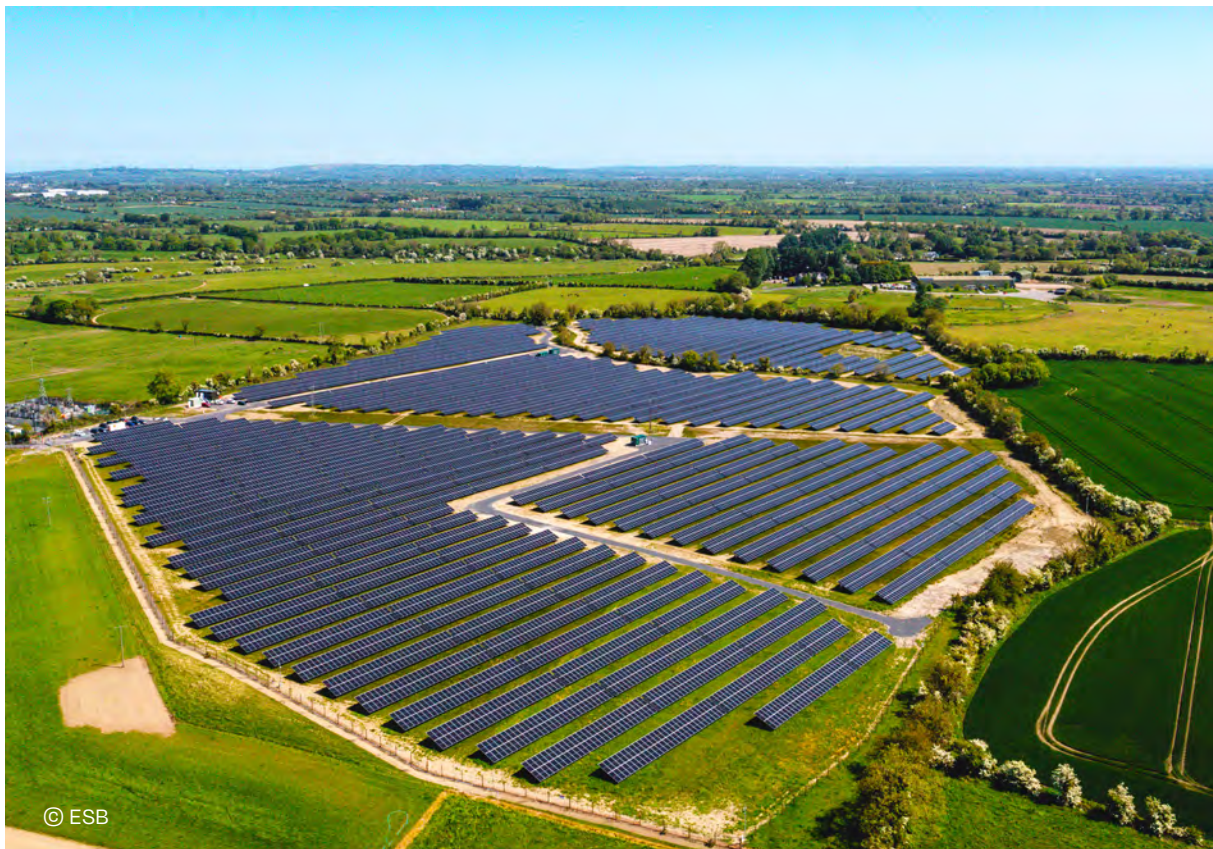
8 MW, Bullstown PV park, Ashbourne, Ireland
