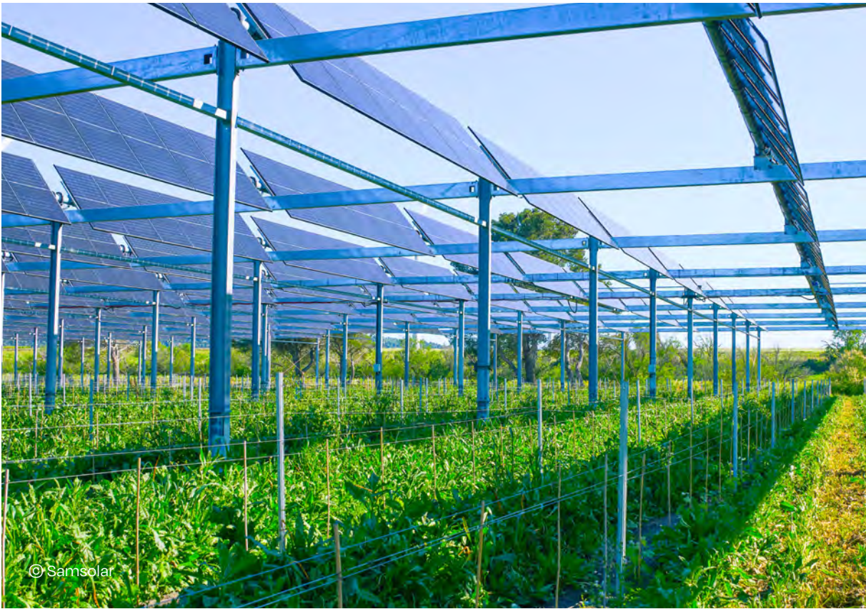
3 MW Agri-PV plant in Cruscades, France.
