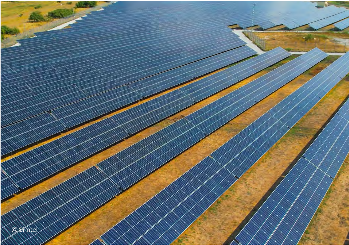
Simtel's 5.5 MW solar park in Salonta, Romania, using Longi PV modules and FIMER inverters.
