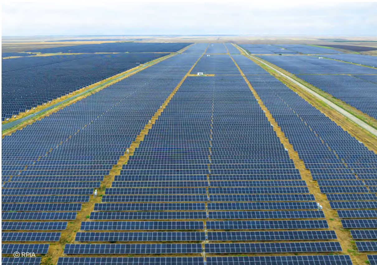
63 MW + 16 MWh BESS, Lumina PV park, Solar Open Day III, Romania.
