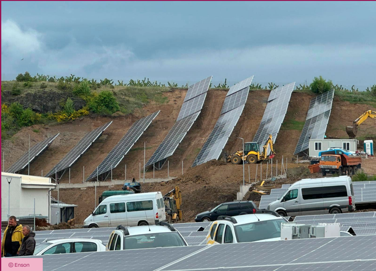
117 MW Konyavo project, Bulgaria
