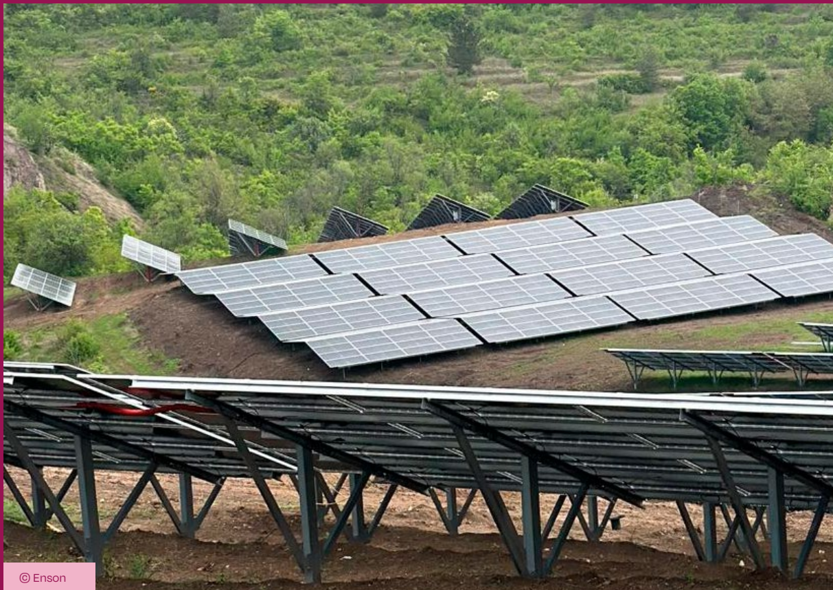
117 MW Konyavo project, Bulgaria
