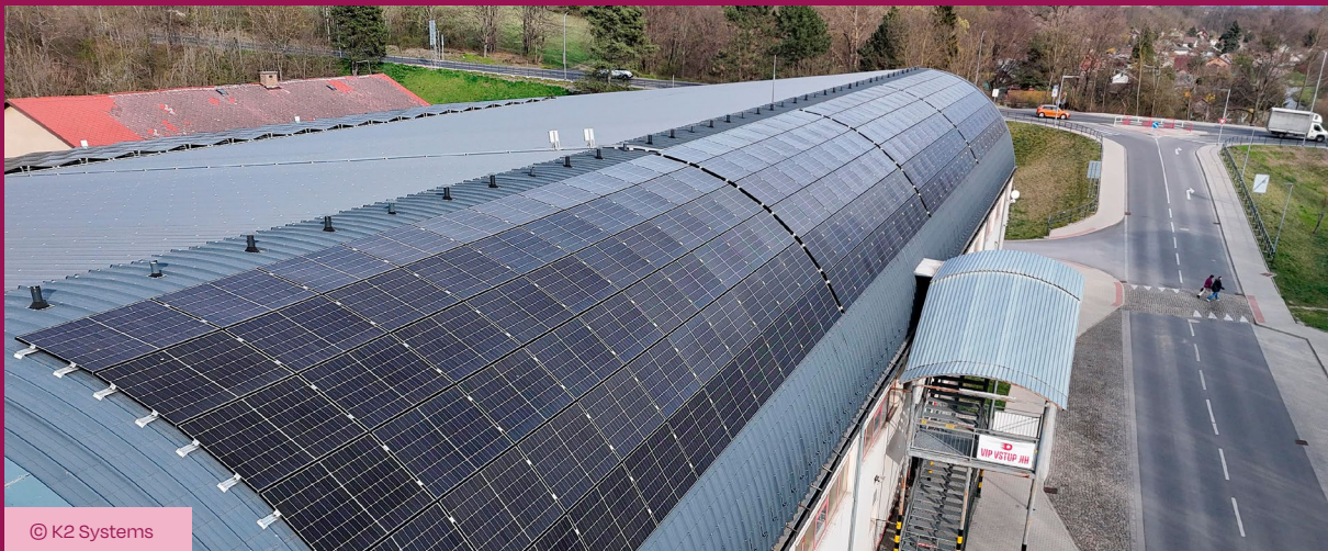
210 kWp rooftop solar, sports facility, Czech Republic
