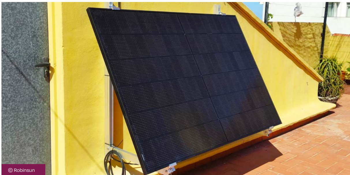
© Robinsun Façade plug-in solar, Valencia, Spain
