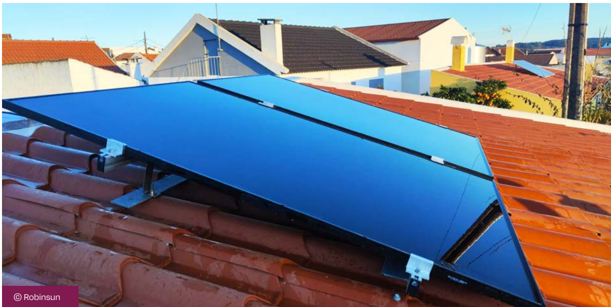
Rooftop plug-in solar, Alenquer, Portugal
