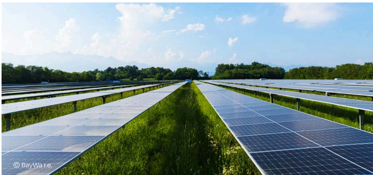
6.5 MW Cerrione solar PV plant, Italy
