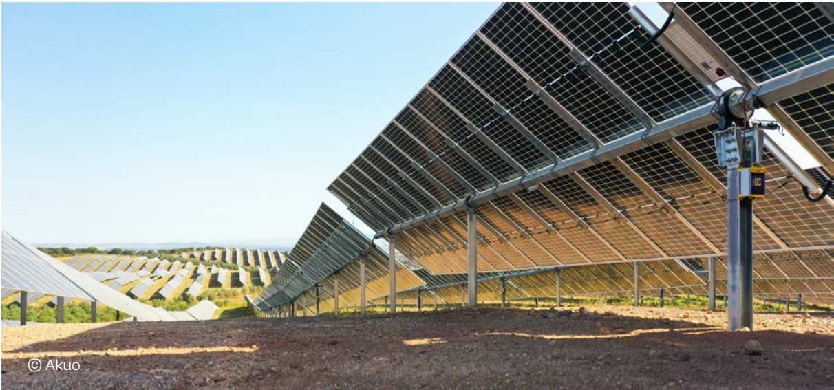
183 MW solar plant, Santas project, Portugal
