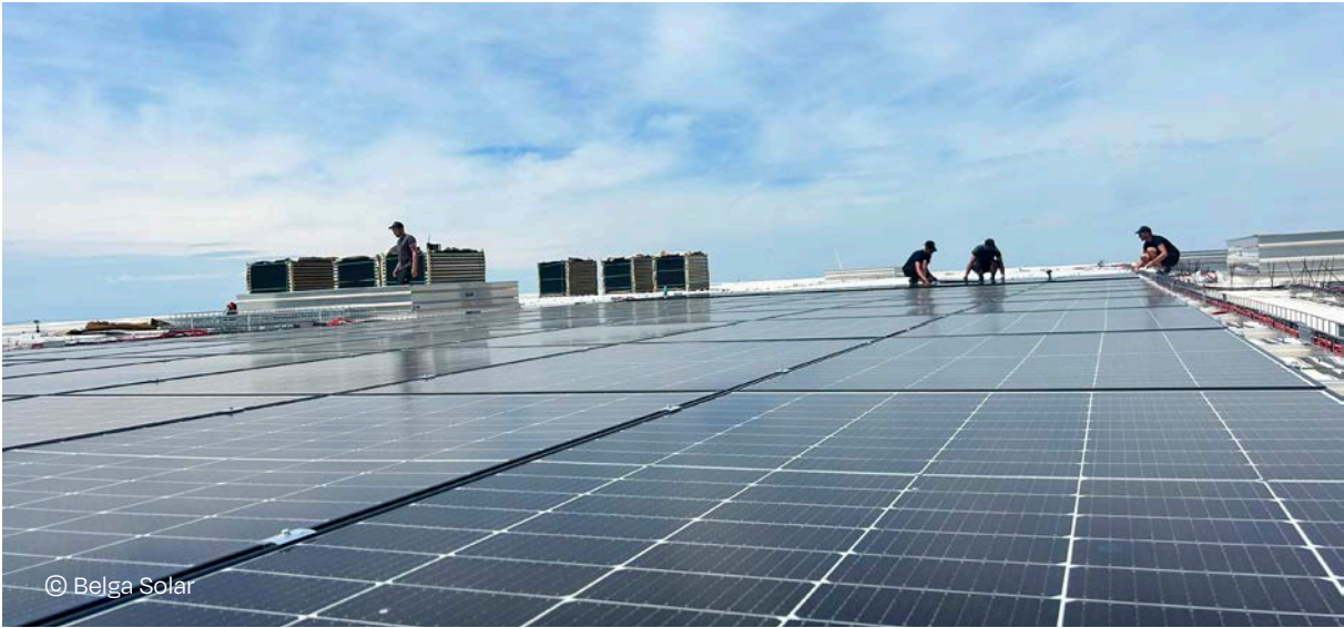
PV installation in Ciney, Belgium
