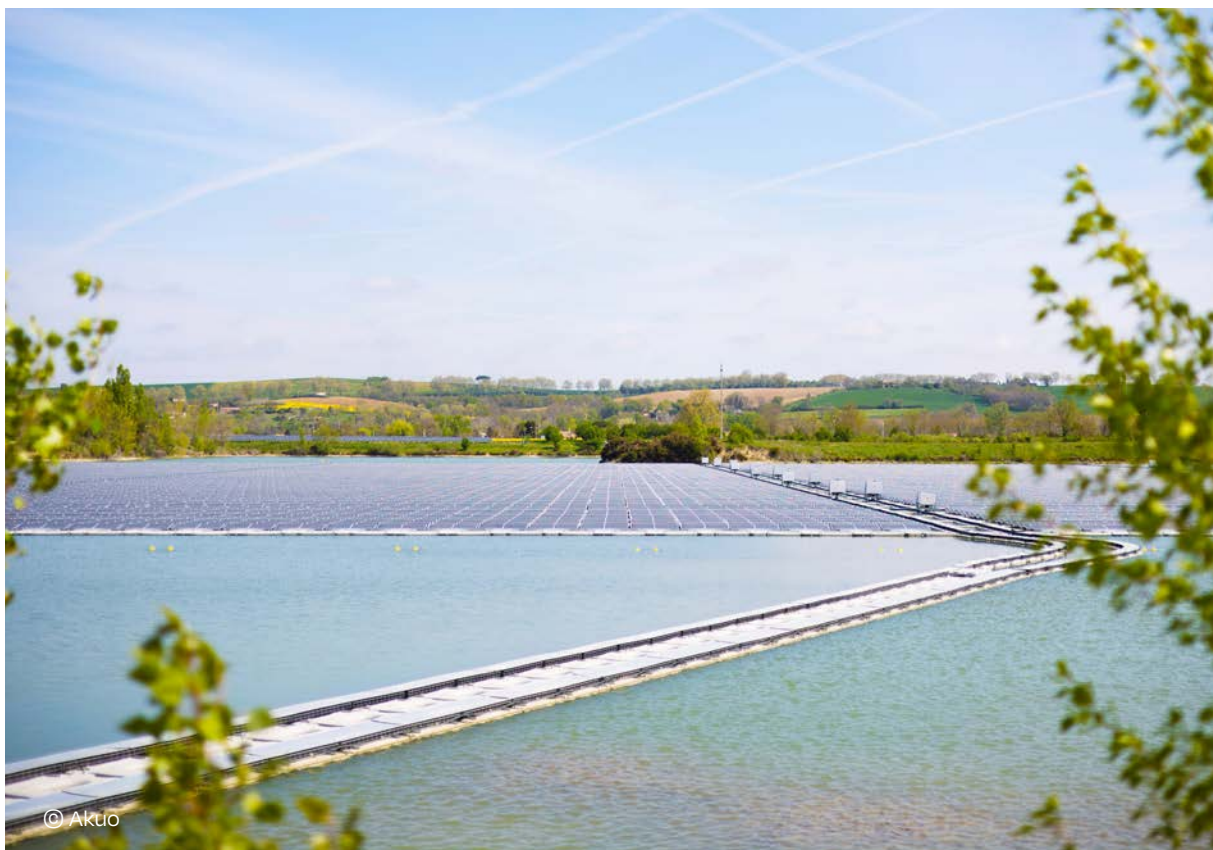
8.7 MW Cintegabelle solar park, France
