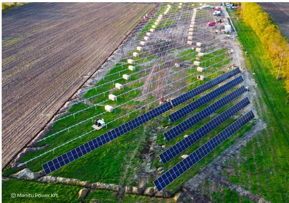
1 MW 1 axis tracker installed PV plant under construction in Komárom-Esztergom County, Hungary
