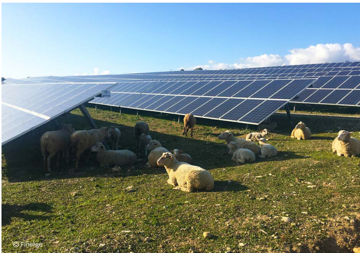
4.5 MW solar project, Faro, Portugal
