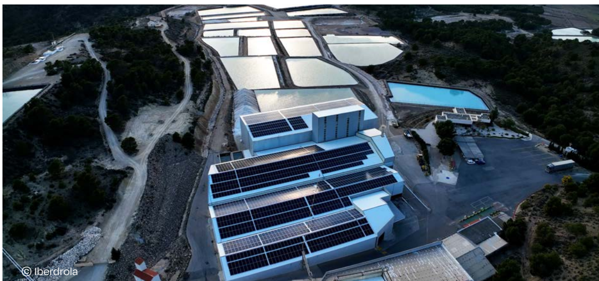
5 MW self-consumption PV plant, salt company Jumsal, Jumilla, Spain.
